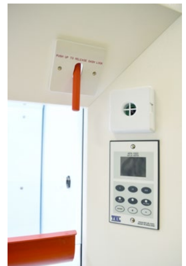
Control panel and sash lock.
